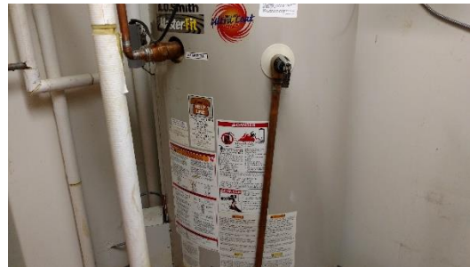
Uninsulated Gas Fired Domestic Hot Water Heater
