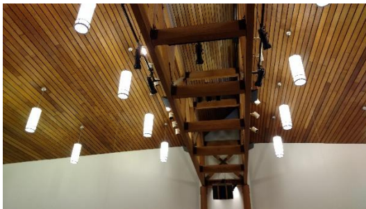
Sanctuary High Bay Spot Lights
